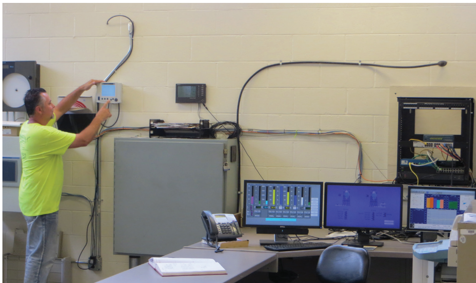
Mahoning County staff checks the settings on the IQ SensorNet 2020 XT Controller
