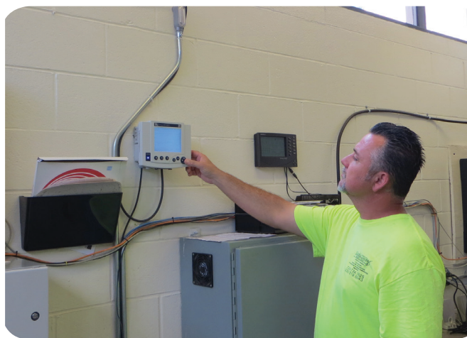
Cappitte checks the settings on the IQ SensorNet 2020 XT Controller
